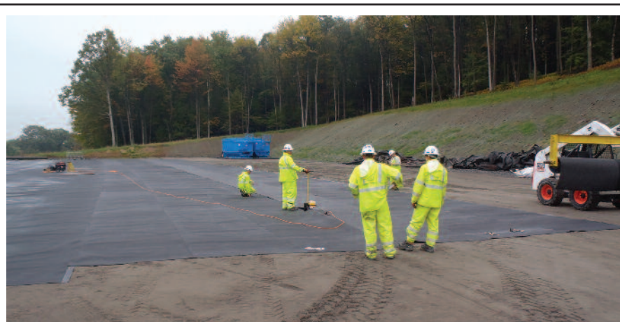
If the top layer of containment sub-base is too hard, protruding debris and stones cannot be pushed down and may result in punctures. If the sub-base is too soft, ruts may cause traffic to bounce and embed equipment forks into the liner.
