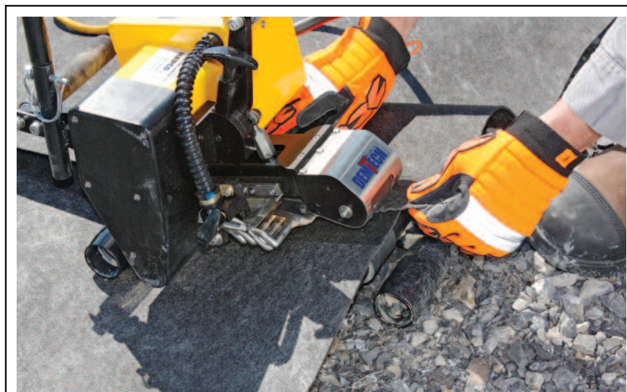
Large liner panels should be seamed together with a wedge welder, rather than a hot air gun or extrusion welder, to ensure good seam contact over long lengths. The welder should be set to the correct temperature and speed, depending on liner and site conditions.
