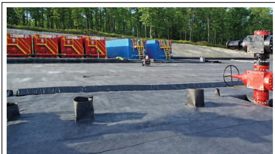
Drilling pad containment typically consists of some local containment deployed around specific contaminant sources such as reservoir, fuel or chemical tanks, along with complete containment deployed over the entire pad. In either case, liners should be durable, impervious, and chemically compatible with the liquid.
